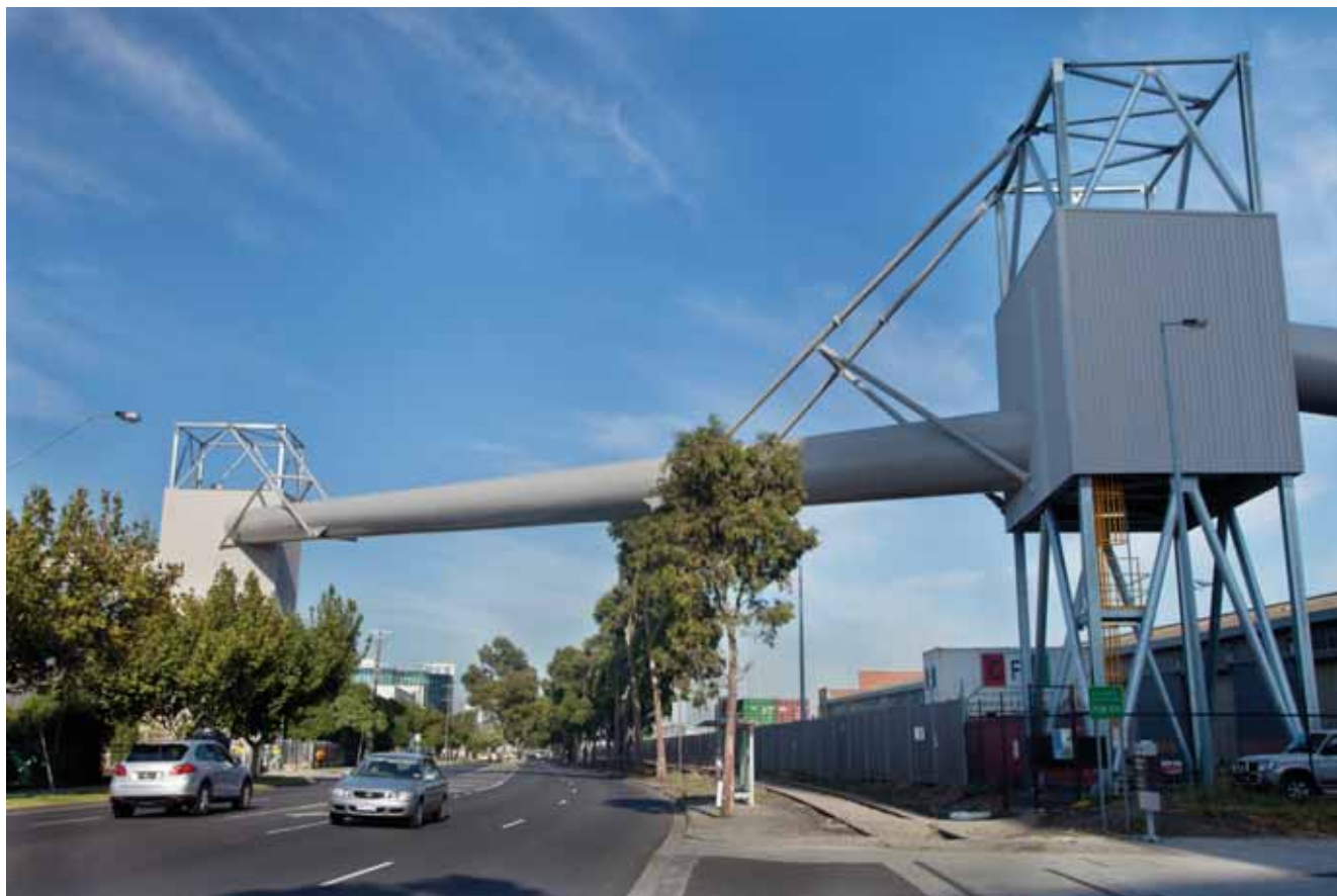
The new Gypsum receiving/conveying system over Lorimer Street, Port Melbourne.
